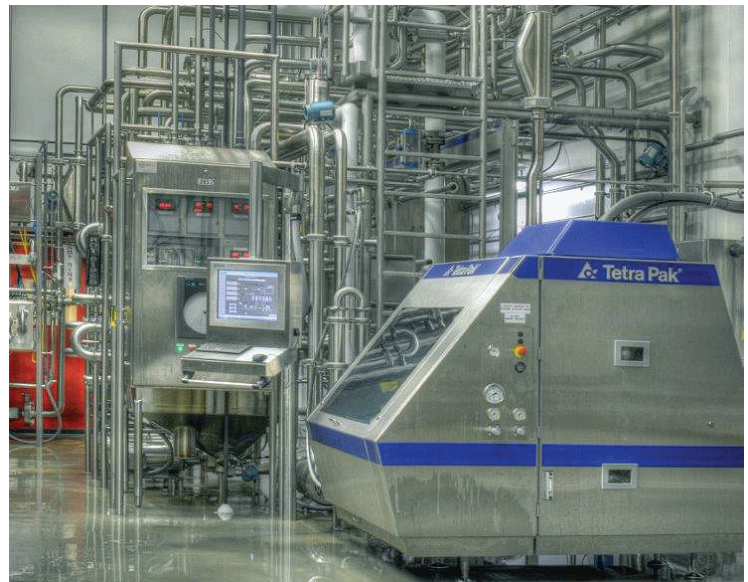
At the Galloway Company, located in Neenah, WI, about 20 miles of two-inch stainless steel piping runs throughout the plant.
